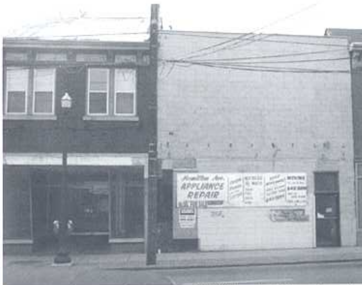
Poor building conditions on 4000 block of Hamilton Ave.
